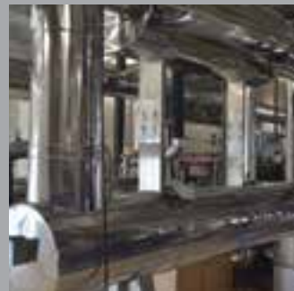
Exhaust Heat Boiler
